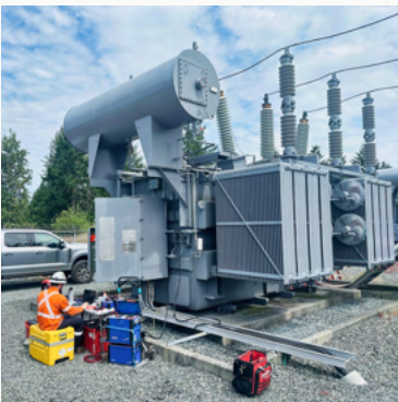
Transformer testing and diagnostics
