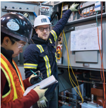
Full-system commissioning verification
